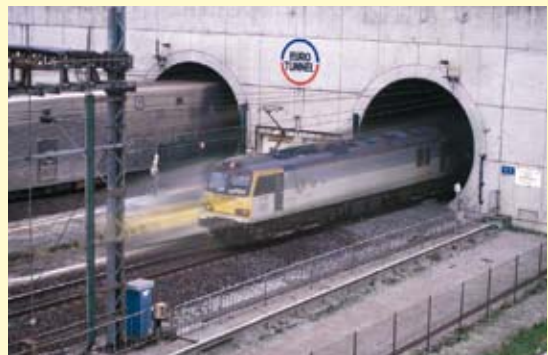
CLIC is often used for cable fixing in railway- and underground tunnels.
