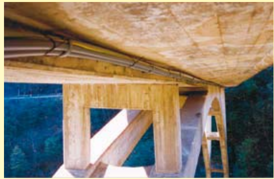
Bundled pipes and cables with one CLIC clamp at the underside of the Ponte Val Calanca bridge in Switzerland.
